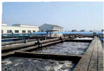
造纸污水处理 Papermaking wastewater treatment
